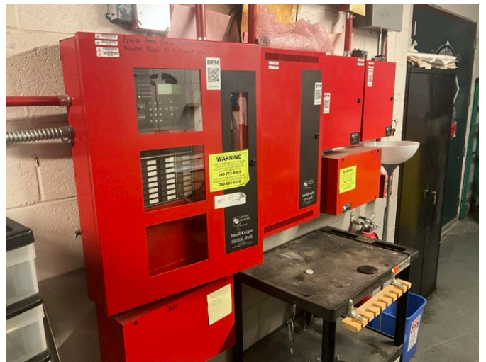
22 - FIRE ALARM PANEL
