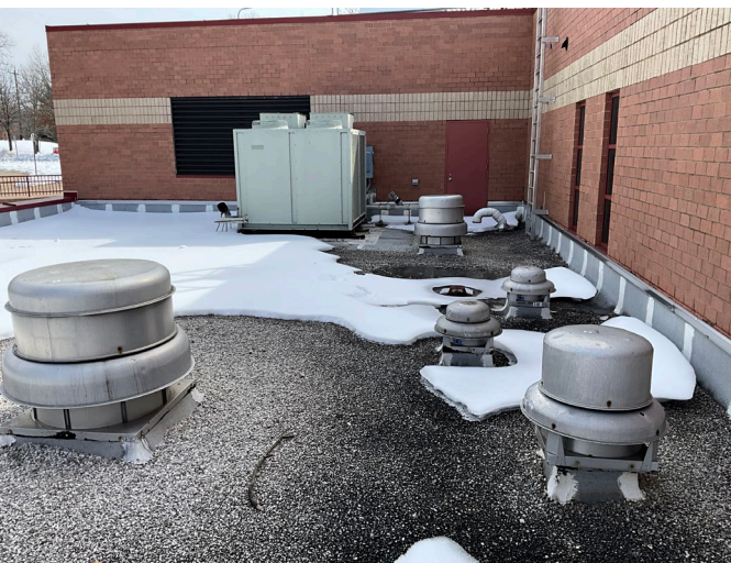
17 - ROOFTOP MECHANICAL EQUIPMENT
