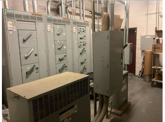
20 - MAIN ELECTRICAL ROOM
