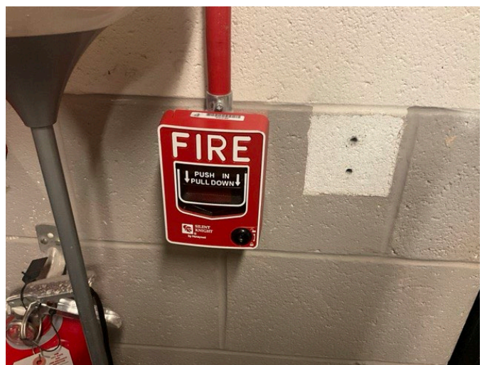
24 - FIRE ALARM DEVICES
